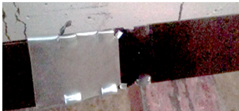
Figure 12: Location of failure in the clip of beam 05.
